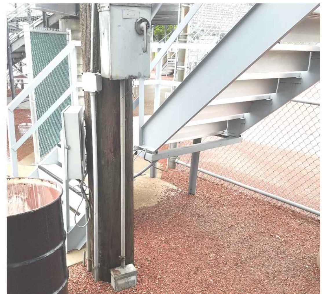
EXISTING ELECTRICAL EQUIPMENT - EAST SIDE
